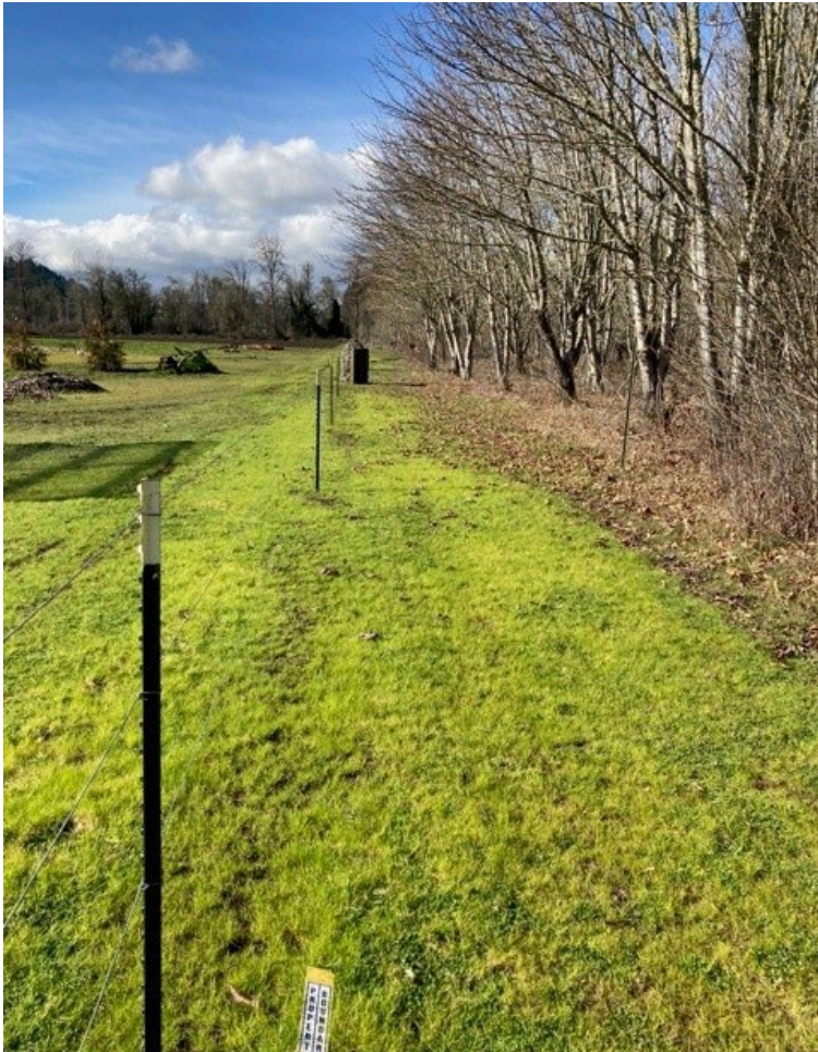
Photo 5. Rock jack style fence being installed on the Sorenson Meadow boundary to protect a culturally sensitive site from damage from trespass. J. Blazar photo.
